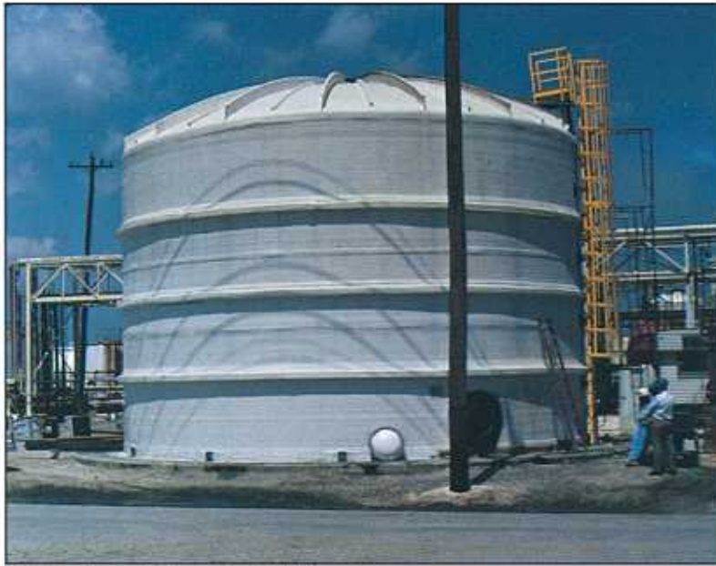
38' Diameter Acid Storage Tank, 1980
