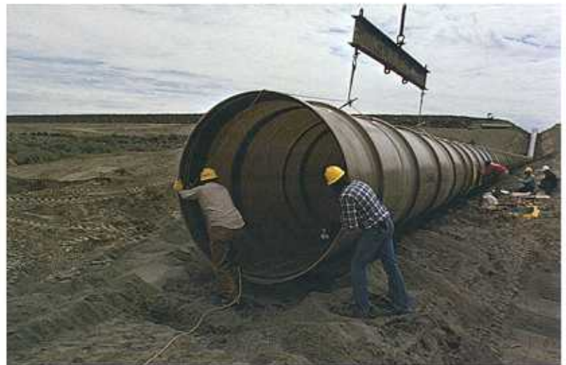
7 ft. dia. buried circulating water pipe
