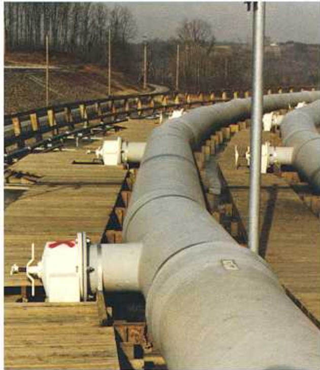
Cooling water distribution pipe
