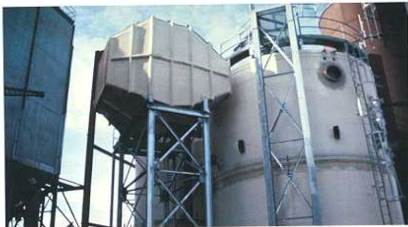
28 ft. dia. FGD reactor/absorber and mist eliminator
