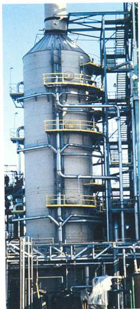
24 ft. dia. absorber tower
